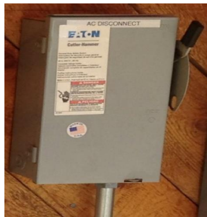
Figure 1.22. Examples of AC safety disconnect switch boxes.
