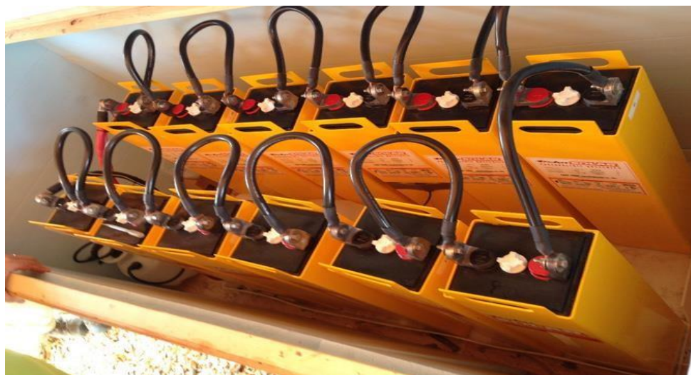
Figure 1.18: A bank of two strings of 2 volt batteries wired in series. Each string is 12 volts
