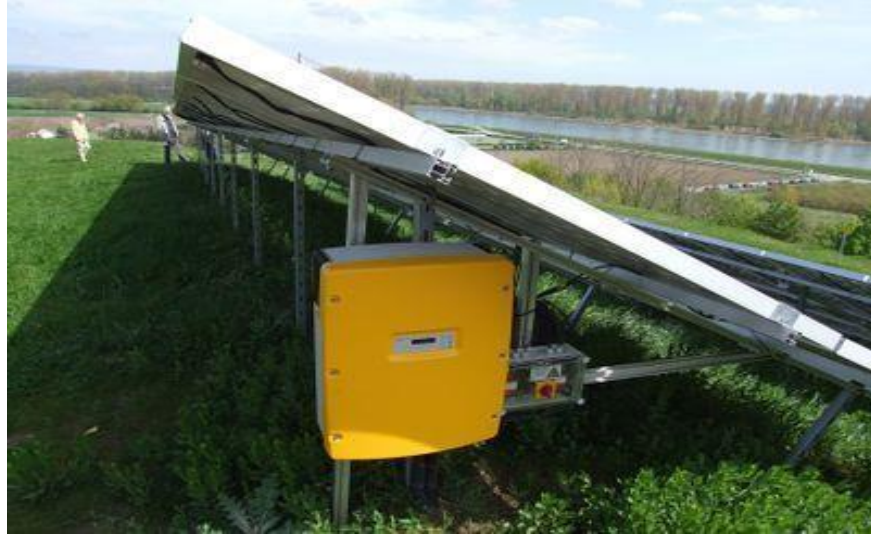
Fig 1.23: solar inverter (yellow) mounted to the solar racking converts DC electricity from the solar array to useful AC electricity
