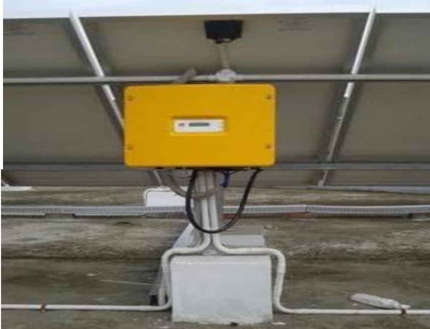
Fig 1.6: Field Junction Box (FJB)
