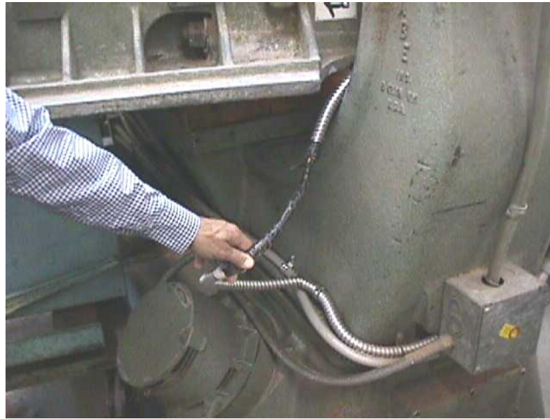
Damaged cord improperly repaired
